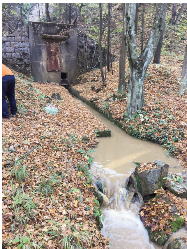
Fig. 5. Muddy, heavily polluted water of the Kaludjerica spring during low water season (December 1 st 2019).
